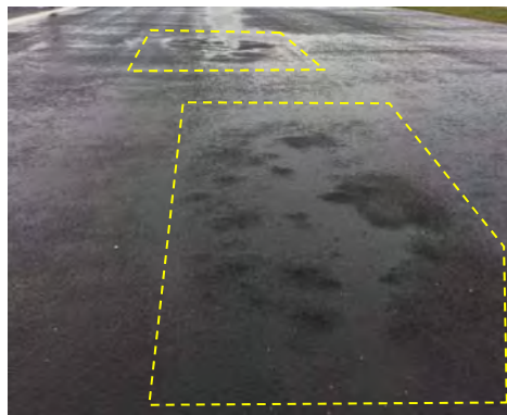
Venting areas can be identified by small bumps in the basecourse. This is most obvious after rain, in evening light or during venting
