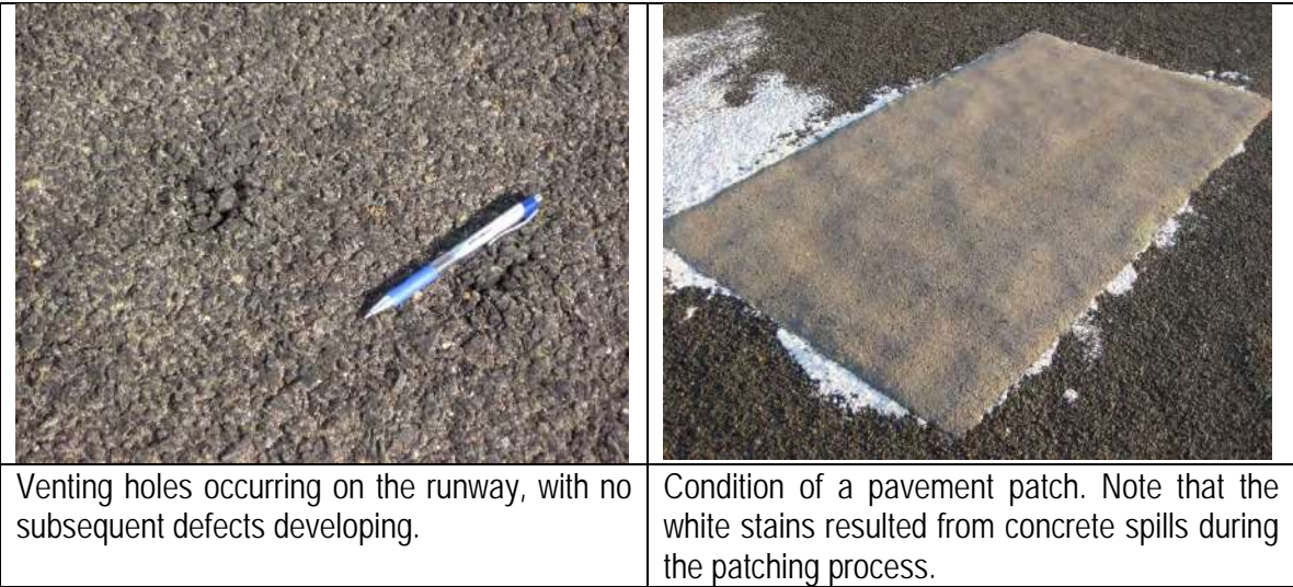
Figure 4.2: Surface Venting Holes and Patching of the Runway
