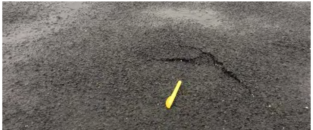
Observed rupture of 3-coat bitumen surface during significant venting (Condition Score = 2)
