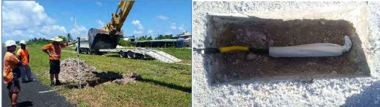
Figure 3.1: -Installation of Piezometer in BH1 and Installation of vapour pressure logger within the shallow pit.
