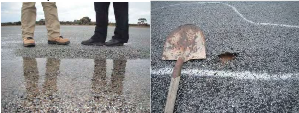
Figure 2.10: Blistering on the Seal at Albany City Airport (Paul G Robertson & Associates, 2011))
