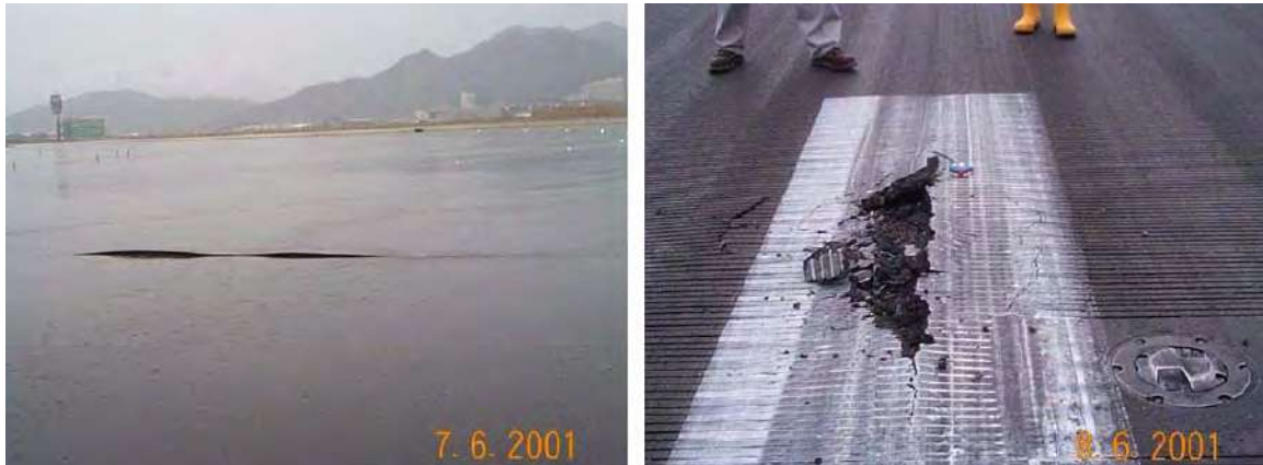
Figure 2.6: Damage on the Hong Kong Runway (Leung et al., 2007)
